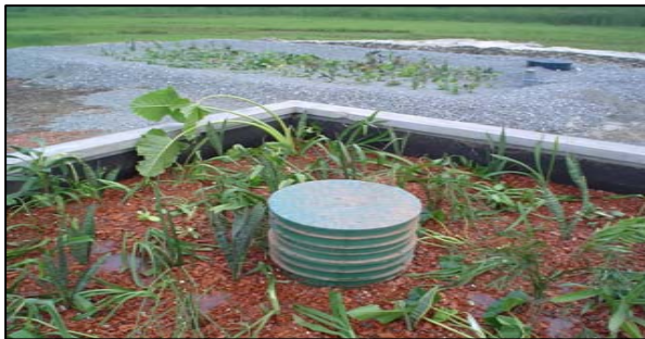
Tema Living Machine newly planted wetland cell
